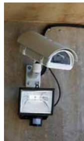
Exterior Security Lighting
