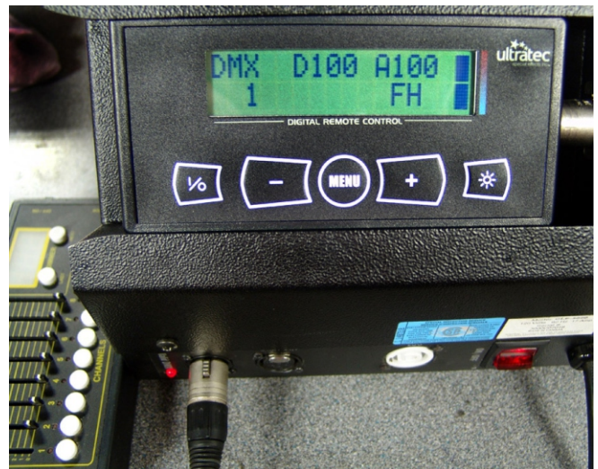
Machine on with DMX. Machine was fully heated (note bar graph) but heater starts for 100% Actual flow.
